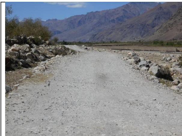
BT washed away at Km 221+100
