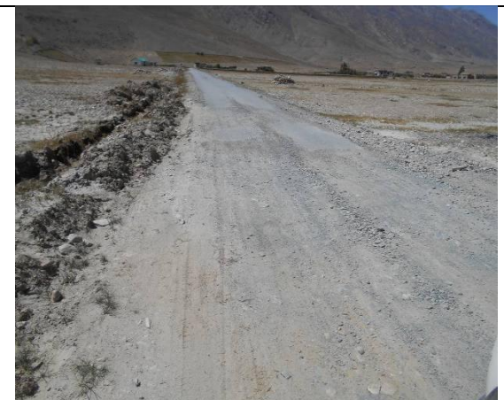
Poor section at Km 230+000
