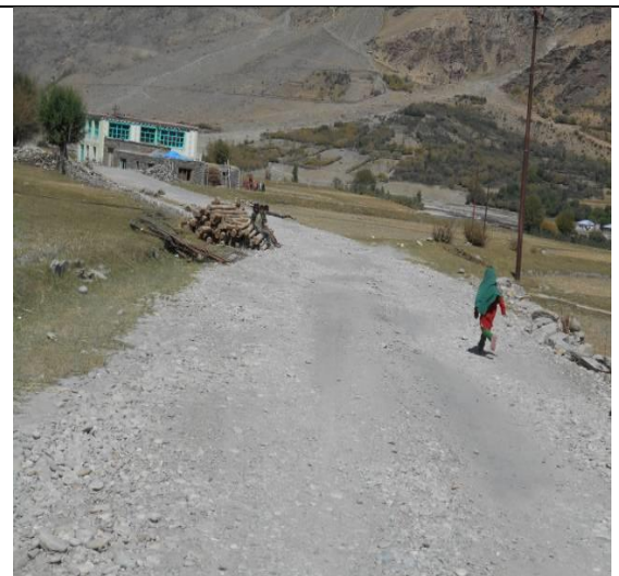
BT washed away at Km 60+800
